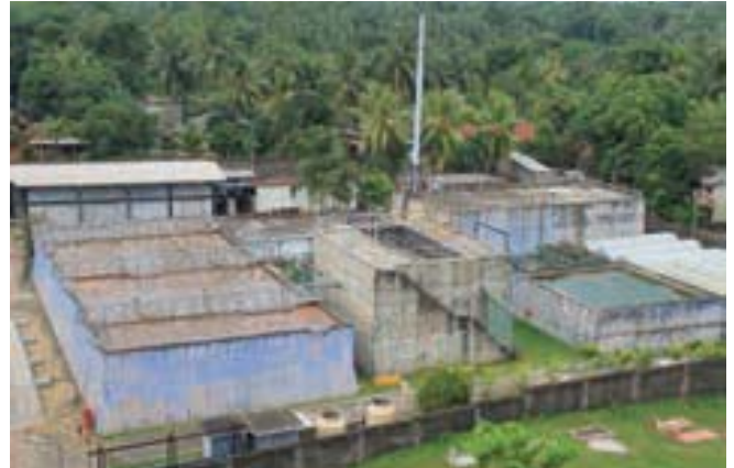
Waste water treatment plant at Biyagama, Sri Lanka
